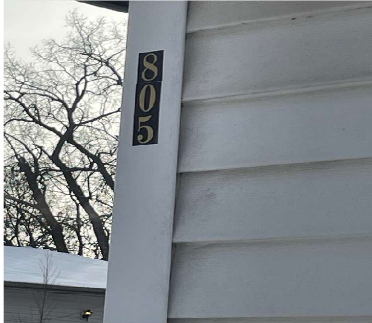
805 Minnehaha Ave W Reinspection on 1/5/2026
